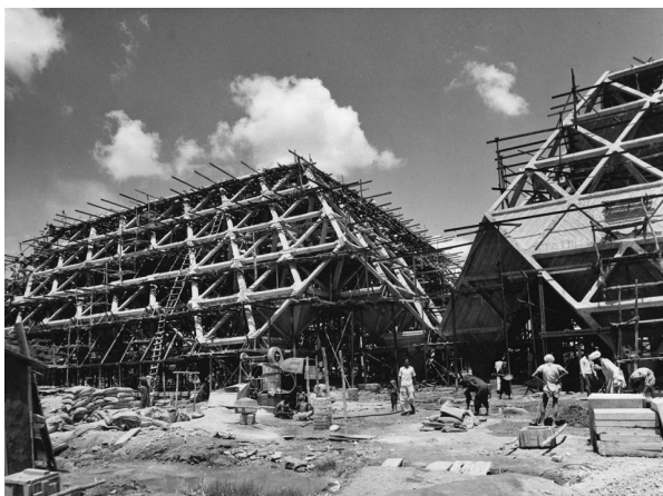
Figure 3.1.1. Halls of Nations and Industries under construction: Space structure was not built in pre-fabricated steel structure but in concrete because of the abundance of available laborers who could fabricate wood formwork and cast concrete on site. This story shows how concrete associates with two conflicting conceptions simultaneously: advanced technology and traditional craft. Raj, Mahendra, and Raj Rewal. Halls of Nations and Industries, Pragati Maidan, New Delhi, India - Reprinted from photograph by Madan Mahatta, architexturez.net/doc/az-cf-181543 , 1972.
