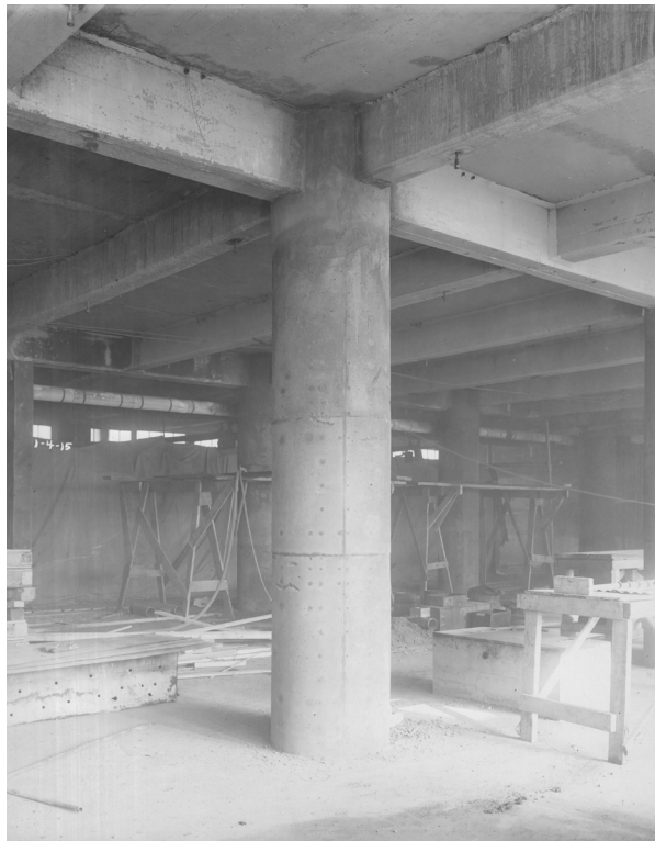
Figure 5.3.6. Edison's column: A concrete column constructed with conventional formwork - Reprinted from Thomas Edison NHP, npgallery.nps.gov, 1915.
