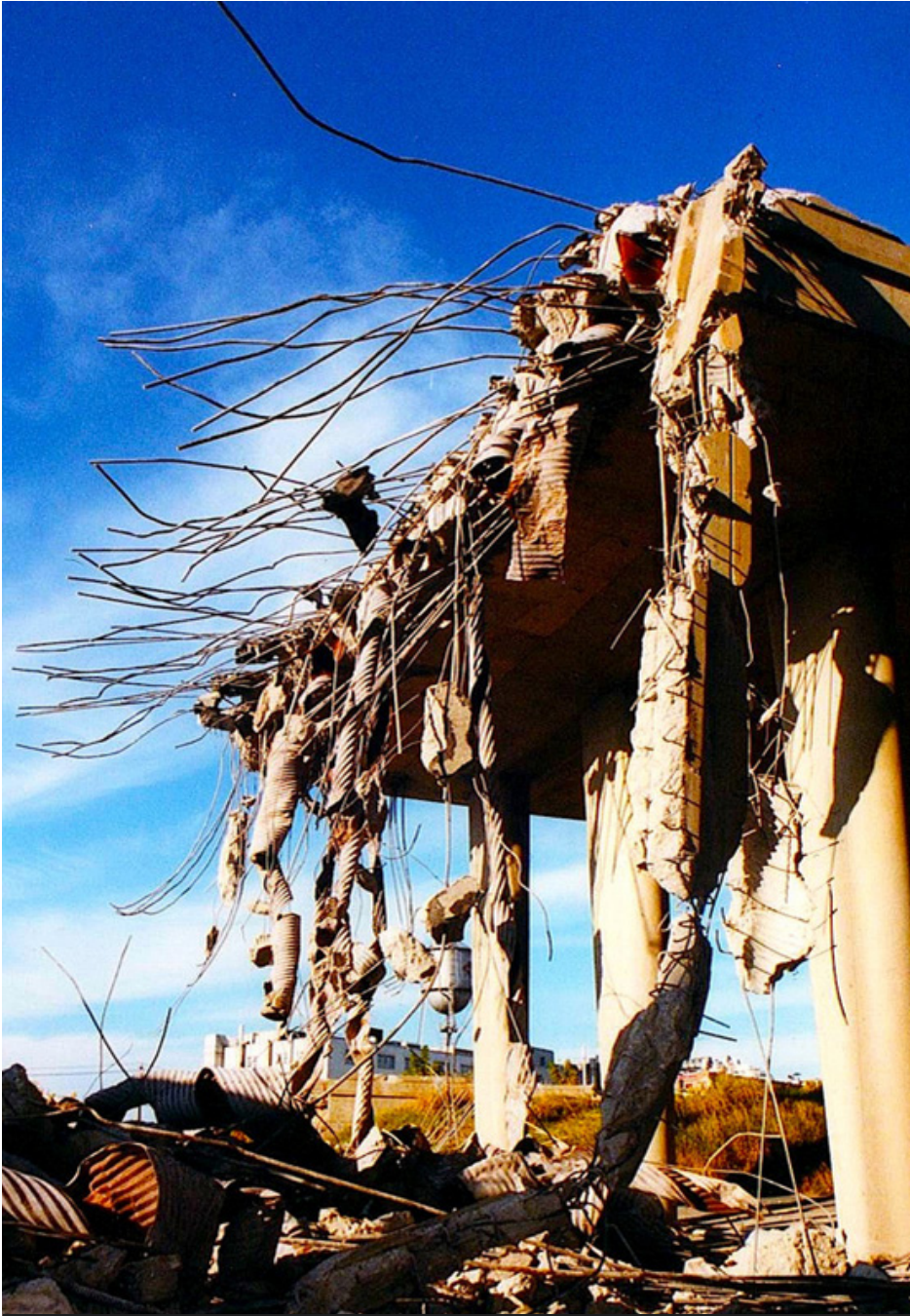
Figure 1: Highway removal in progress in Portland, OR (Reclaiming Old West Broad Street)
