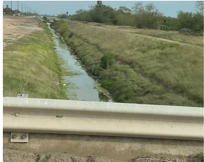
A nearby drainage canal that overflows during rainstorms.
