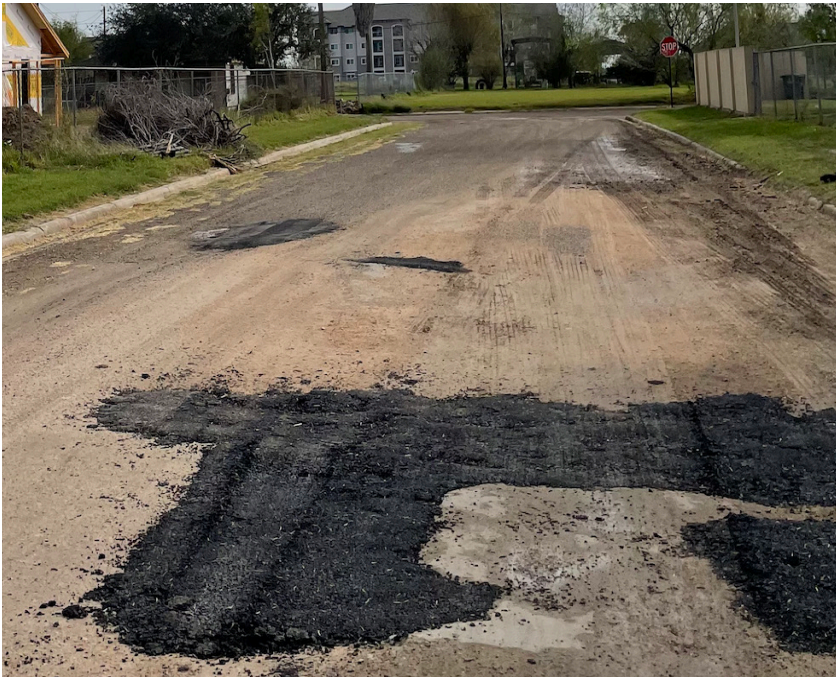
Grassroots pot-hole filling in Alberta Estates #2.
