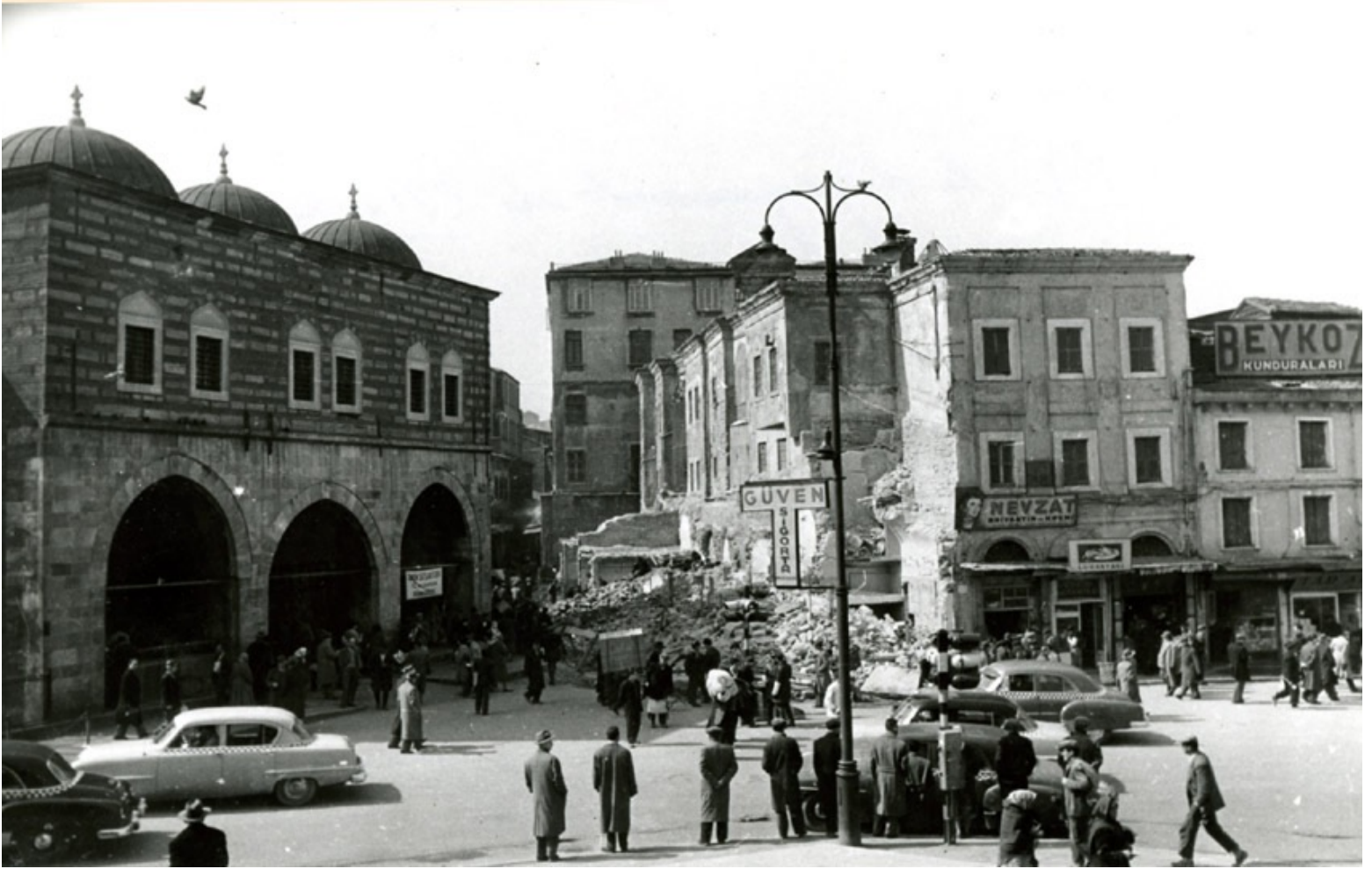
Figure 34 – View of the Eminönü Square site being demolished, undated photograph, Development plan for the Eminönü – Mahmut-Paşa – Divan Yolu area, 1943–1944, from Académie d’architecture, Cité de l’Architecture et du Patrimoine, Archives d’architecture du XXe siècle, Fonds Henri Prost, 343 AA 67/1.
