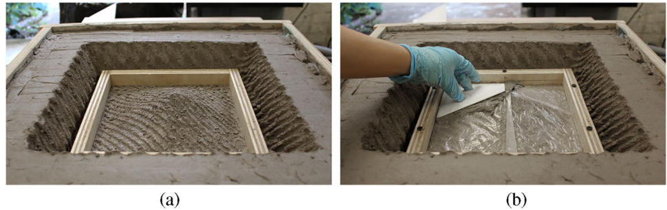
Fig. 19 (a) Vertical timber members added to perimeter of adobe formwork, and (b) thickness of first layer of concrete being checked with 3D printed template
