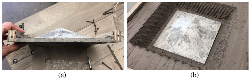
Fig. 21 (a) Side view of cured concrete shell foundation, and (b) cured concrete shell foundation on adobe formwork
