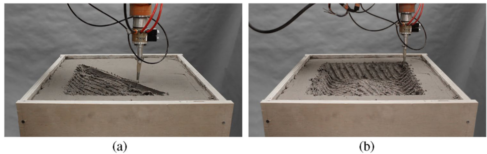
Fig. 17 Robotic milling of adobe to act as formwork for thin concrete shell (a) roughing pass one, and (b) roughing pass three
