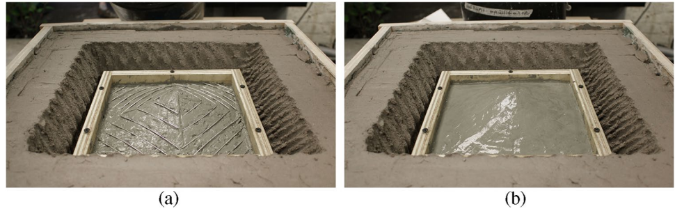
Fig. 20 (a) Rebar added along principal stress lines, and (b) second layer of concrete applied to adobe formwork
