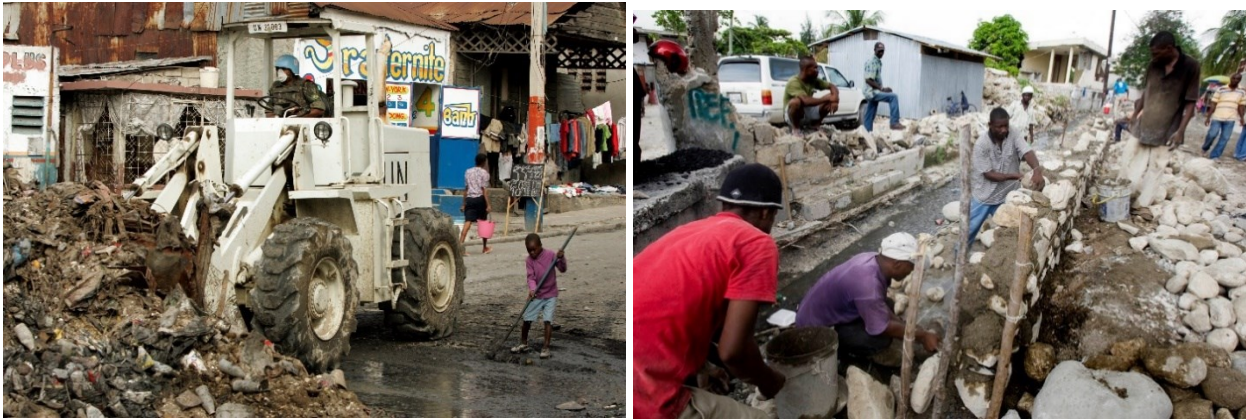
Figure 4.3. MINUSTAH engaged in waste removal in the Bel-Air neighborhood of Port-au-Prince, and employed men from the community to build a canal in Port-au-Prince to improve drainage for the upcoming rainy season as part of the Community Violence Reduction project. Source: United Nations, 27 January 2005, https://www.flickr.com/photos/minustah/34869718066/ (left), https://www.flickr.com/photos/minustah/4875800461/ (right)
