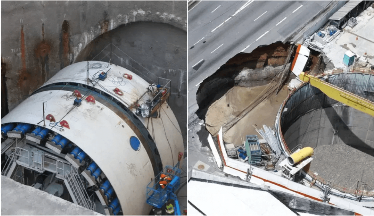
Figure 4-1: Images showing an accident that occurred in the construction of a new metro line in Sao Paulo, Brazil. The accident was caused by unforeseen geological conditions encountered by the TBM (left-hand side) during tunnel construction. A slight course modifications led by adverse ground conditions along the original tunnel line, made the machine's vibration felt on the surface, collapsing a nearby highway and bursting sewage pipes [Garcia, 2022].
