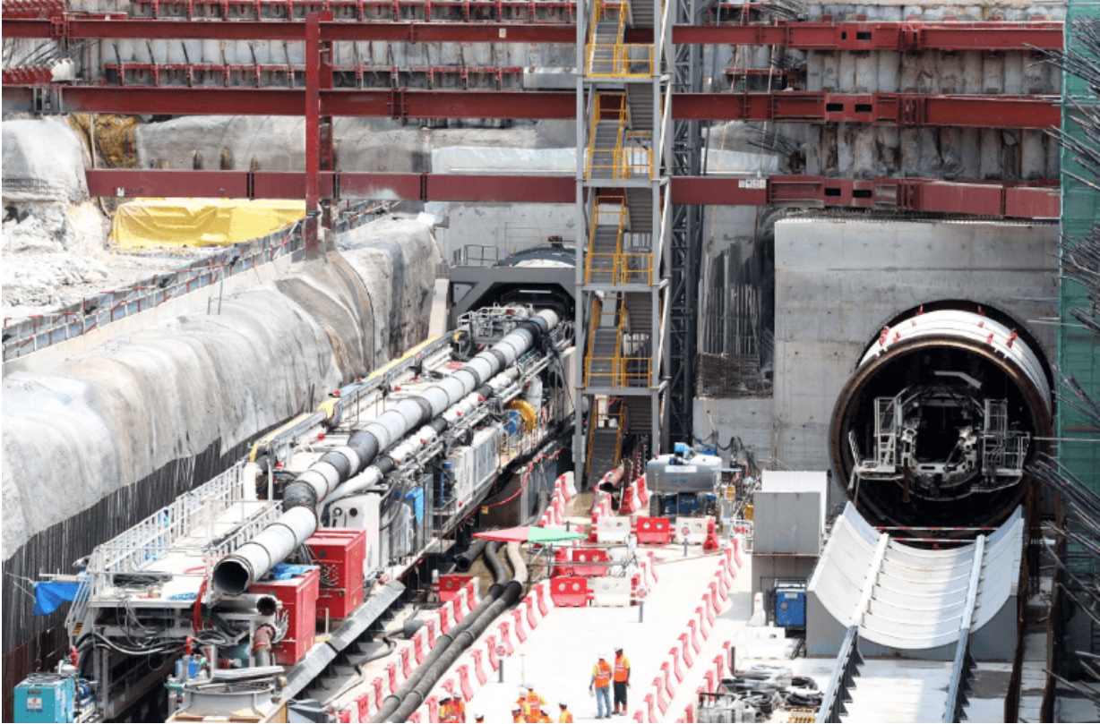
Figure 4-5: Image of the ATBM being setup in a large public transport infrastructure construction site in Malaysia, 2018 [Byrd, 2016]).
