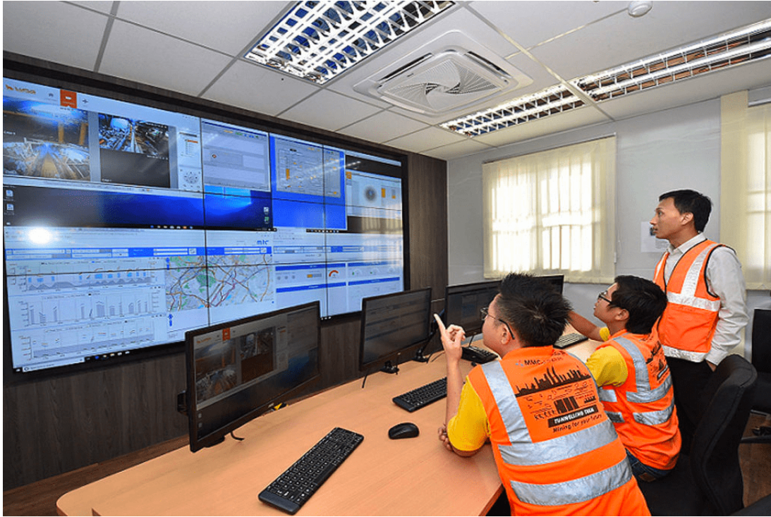
Figure 6-1: Picture of MMC Gamuda's Tunneling Centralized Command and Control Center [Berhad, 2020]).
