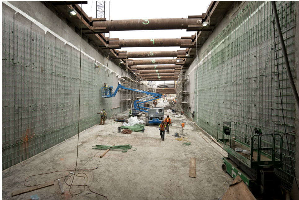
Figure 2-13: Section of the SR 99 tunnel, built through the cut-and-cover method. Seattle, 2015 [Washington State Department of Transportation, 2020].
