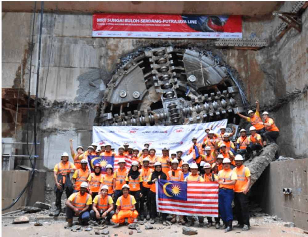
Figure 6-4: MMC Gamuda's A-TBM on the site of the Klang Valley Mass Rapid Transit (KVMRT), using Herrenknecht hardware [Construction, 2021]).
