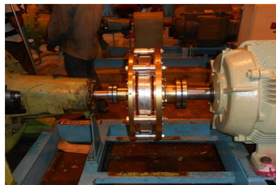
(f) Photo [7] of a magnetic coupling (with its protective shroud removed) driving a ~120 kW water pump at a power plant.
