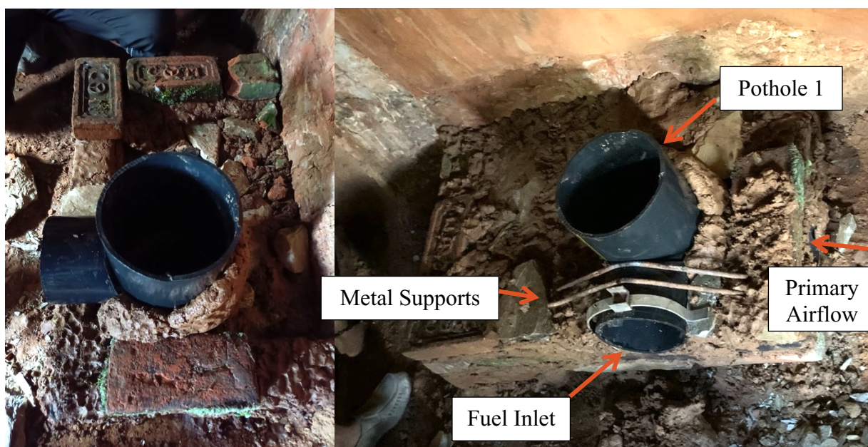
Figure 36: Combustion chamber and fuel inlet PVC pipe molds and brick-clay foundation of the stove
