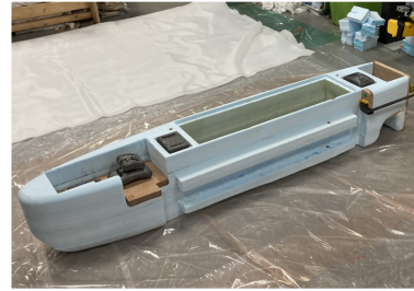
2. Stacking and gluing the foam; installing the wooden inserts using weights and clamps
