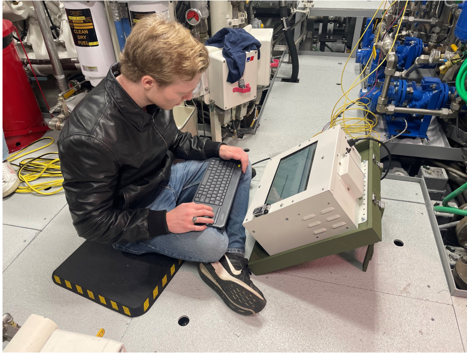
Figure 4.21: Porta-NILM being used to assess the ICCP system.
