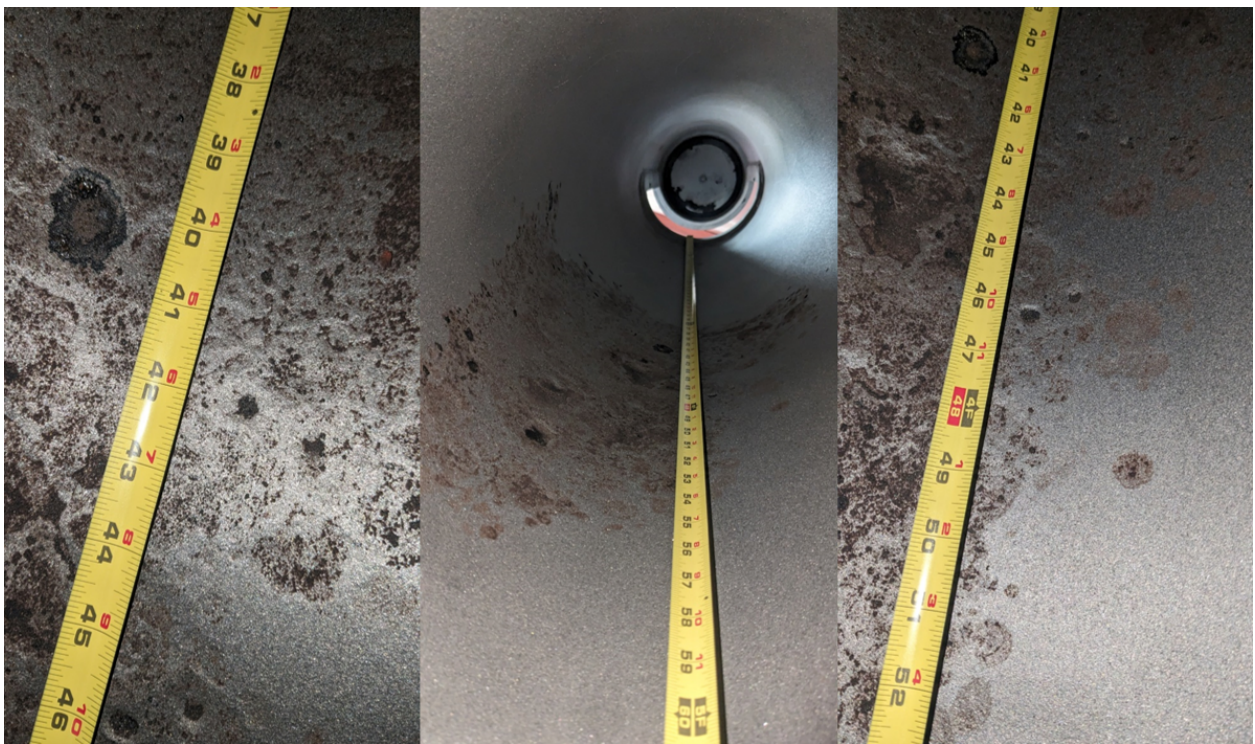
Figure 2.4: Damage to the stern tube of USCGC Charles Moulthroppe after sandblasting[24].
