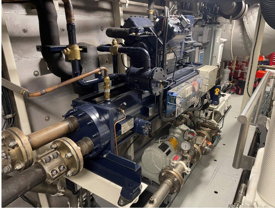
Figure 4.5: Air conditioning compressor C1
