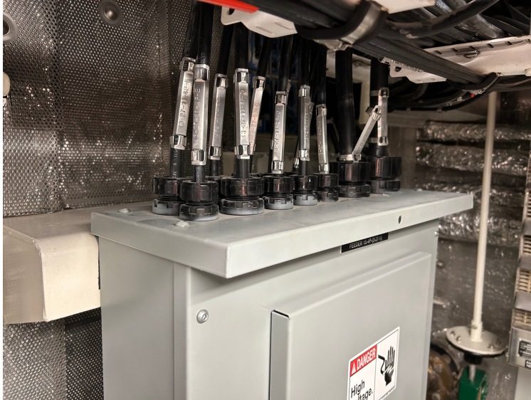
Figure B.9: Cable entries into the top of STBD Machinery Panel (3-27-1).
