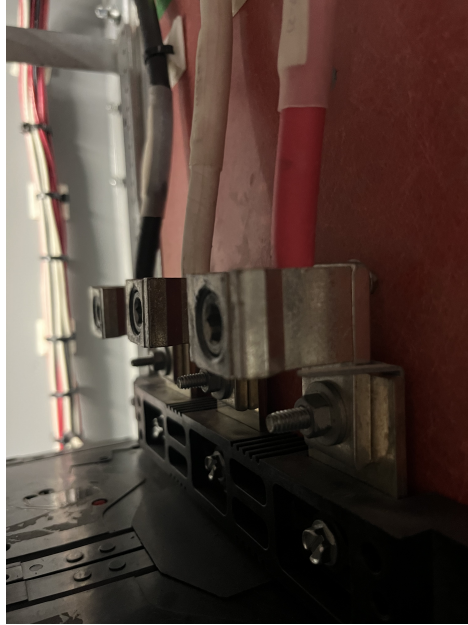
Figure B.13: USCGC WILLIAM CHADWICK (WPC 11050) Power Panel Interior
