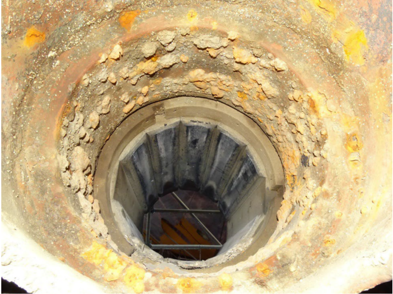
Figure 2.2: Corrosion damage in the stern tube of USCGC Richard Dixon as discovered in dry dock.
