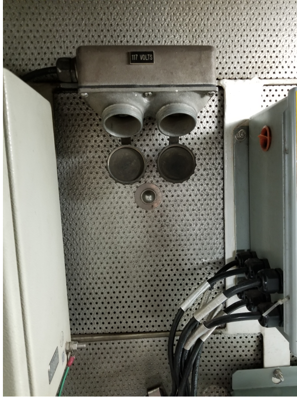
Figure B.7: Power outlet for IEC Cords.
