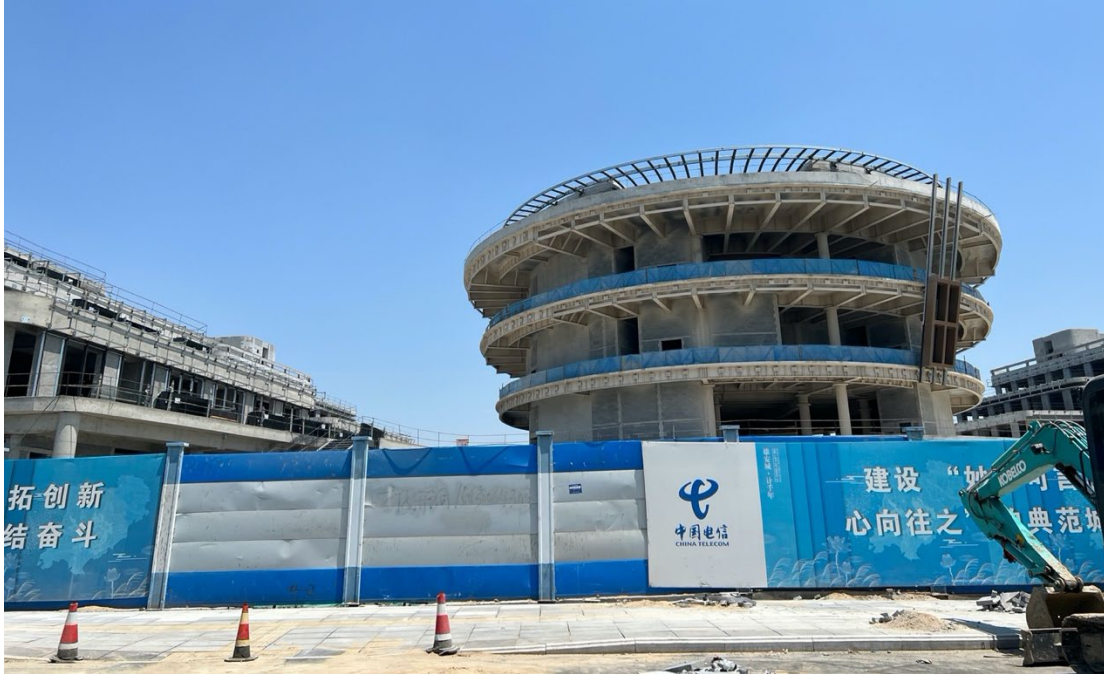
Figure 32a. (above) China Telecom Smart City Research Park under construction, Xiong'an (Author, July 2023)
