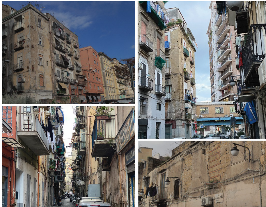
Fig. 38 – Pre-nineteenth-century tuff-made buildings in precarious structural conditions. Pre-nineteenth-century tuff-made buildings in precarious structural conditions. The images were taken by the author during his site visits to the water-facing neighborhoods of Naples. Photos by author (December 2022).
