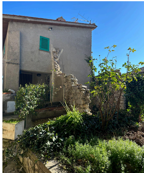
Figure 9: An image of a collapsed structure turned into a garden in Capranica Prenestina. Capranica Prenestina is the biggest town of Monti Prenestini by volume, but also sees some of the most abandonment and physical deterioration.
