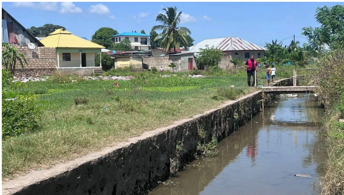
Figure 28 Lack of drainage system increases the susceptibility to flooding in Nyerere
