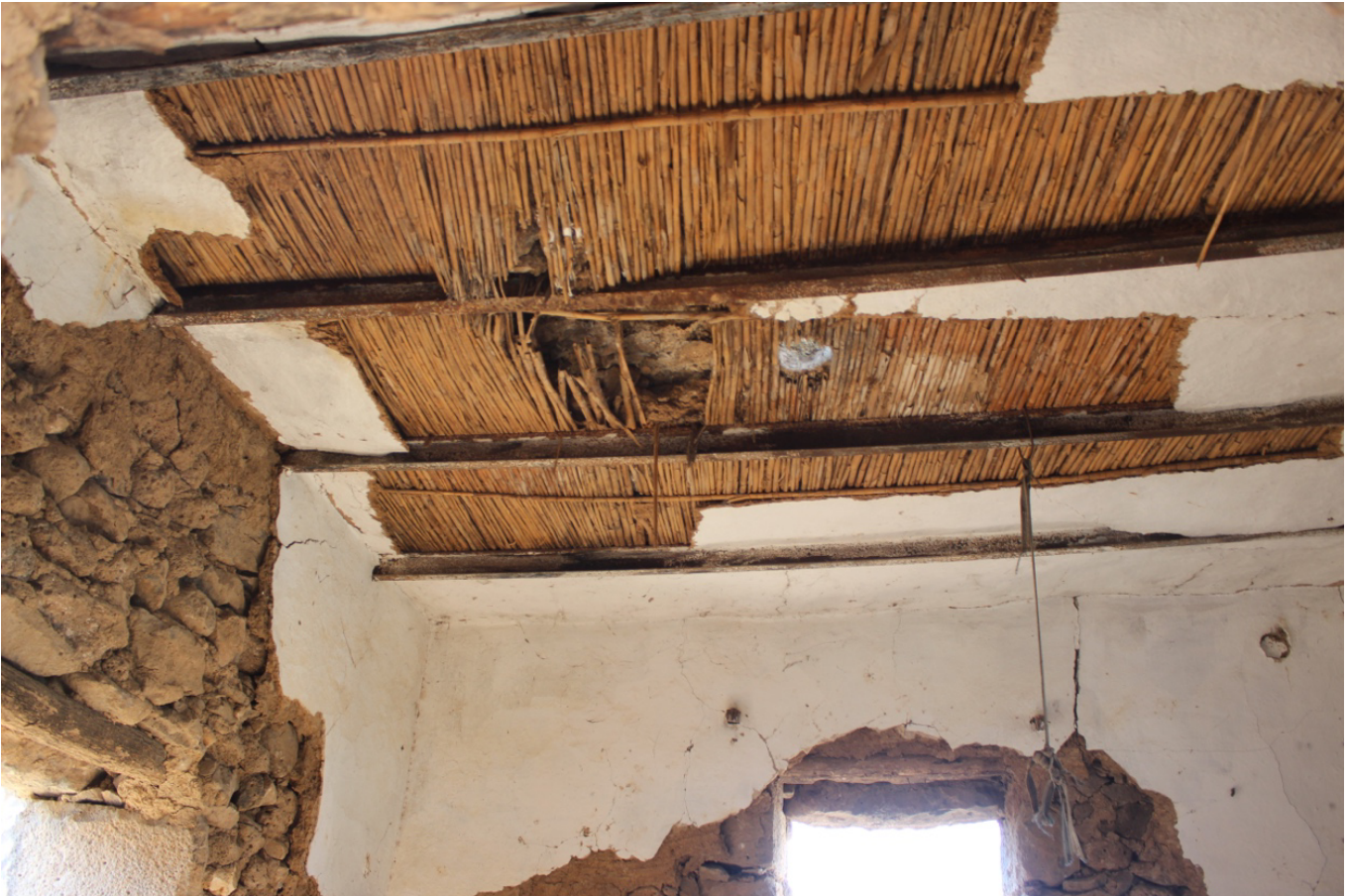
Fig 42. Alali's Crumbling Roof, Nasib, 2021.
