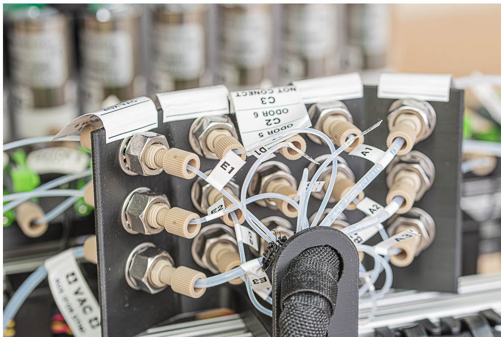
Figure 3.14: Each of the 15 fluid lines in the system umbilical is connected, on the cart side, to another bulkhead panel. Photograph \frac{1}{4} "-28 bulkhead panel at the proximal end of the umbilical where the fluid lines are bundled at the stimulator cart.
