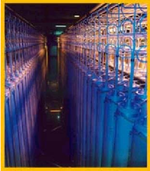
FIGURE 4-3: Centrifuge Enrichment Facility 3 . The photo shows a typical centrifuge enrichment cascade.
