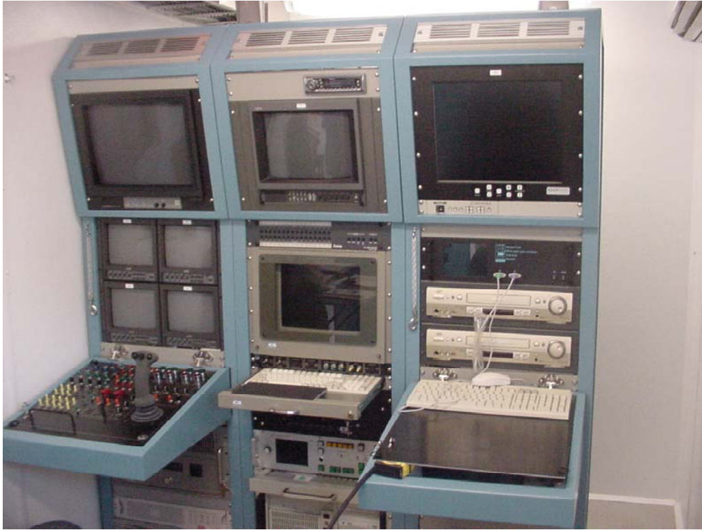
Figure 6. ROV Control Consoles in a Typical Arrangement
