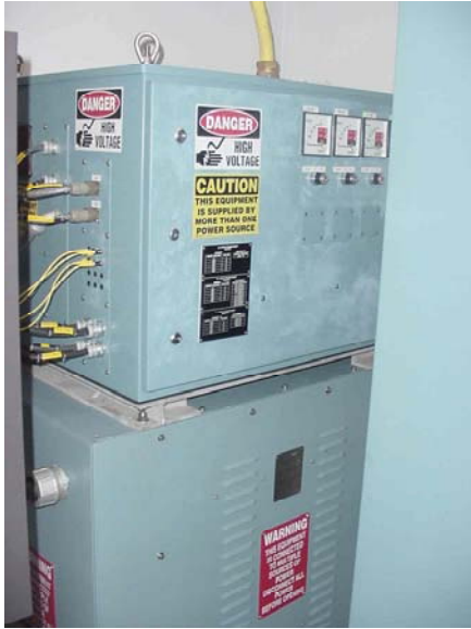
Figure 7. High Voltage Transformer Unit and High Voltage Junction Box
