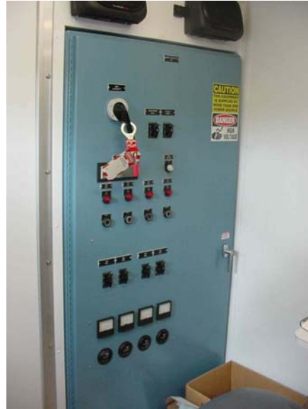
Figure 8. Power Distribution Unit
