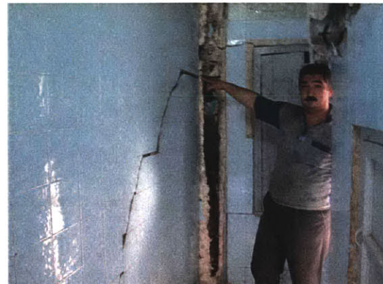
Figure 12. Foundation damage to private home as a result of inadequate water and sewer infrastructure
