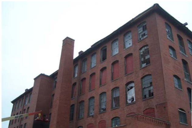
The Bayley Street Lofts is a 25 unit artist live/work project under construction in Pawtucket, RI.
