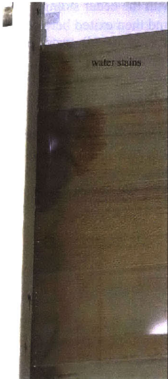
Figure 2-22 Test 4 water stains along the window jamb edge
