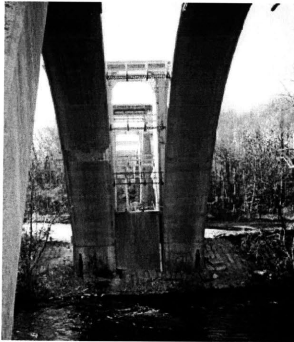
Figure 19. Cumberland, Rhode Island bridge with deck removed. Source: Davis et. al. 2001.
