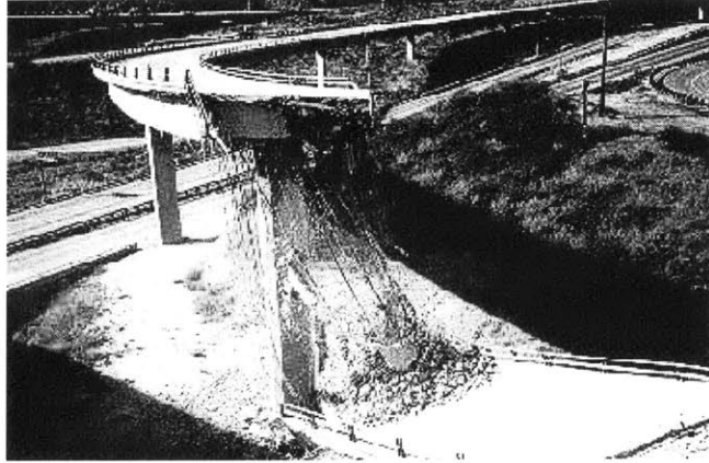
Figure 2-3: Span collapse resulting from complete column failure.
