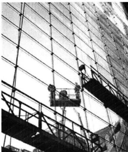
Figure 22: Cable net wall of Columbus Circle, NY
