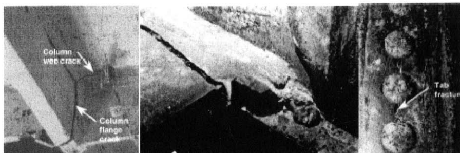
Figure 31: Brittle Steel Connection Failures (Houghton & Karns)
