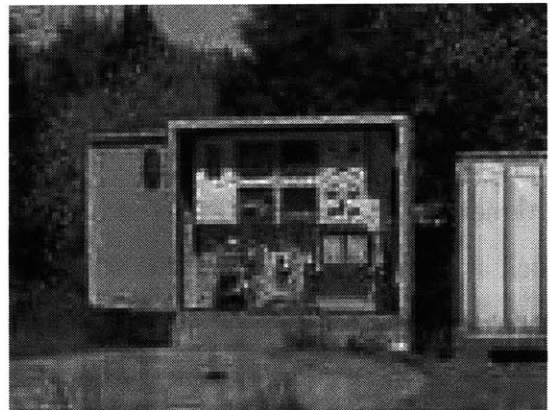
Figure 14: Outdoor Pump Control Panel
