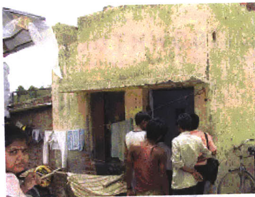
Figure 1: Cement structure in which water pump at the top of the hill is located
