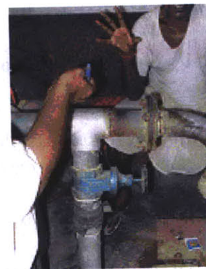
Figure 2. Water pump at the top of the hill
