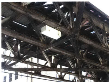
STEEL STRUCTURES IN POOR REPAIR
