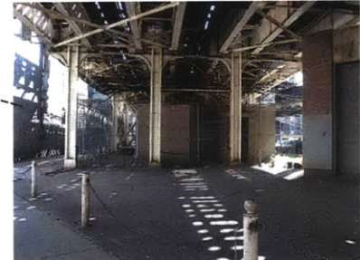
UNACCESSIBLE SPACE OCCUPIED BY COLUMNS, A SUBSTATION, AND A FACILITY
