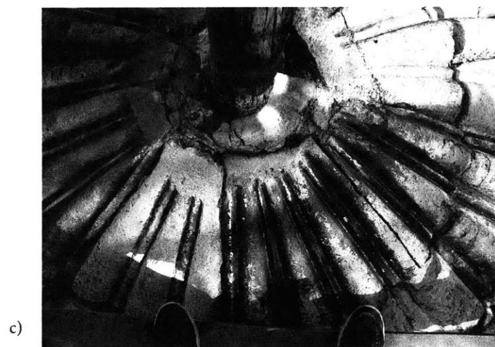
Fig. 2.5 Restoration work at the Mausoleum of Umm Sultan Sha'ban, picture of the second dome, the small one. The pictures show a detail of the same system of wood post holding the crescent in the dome upper part.
