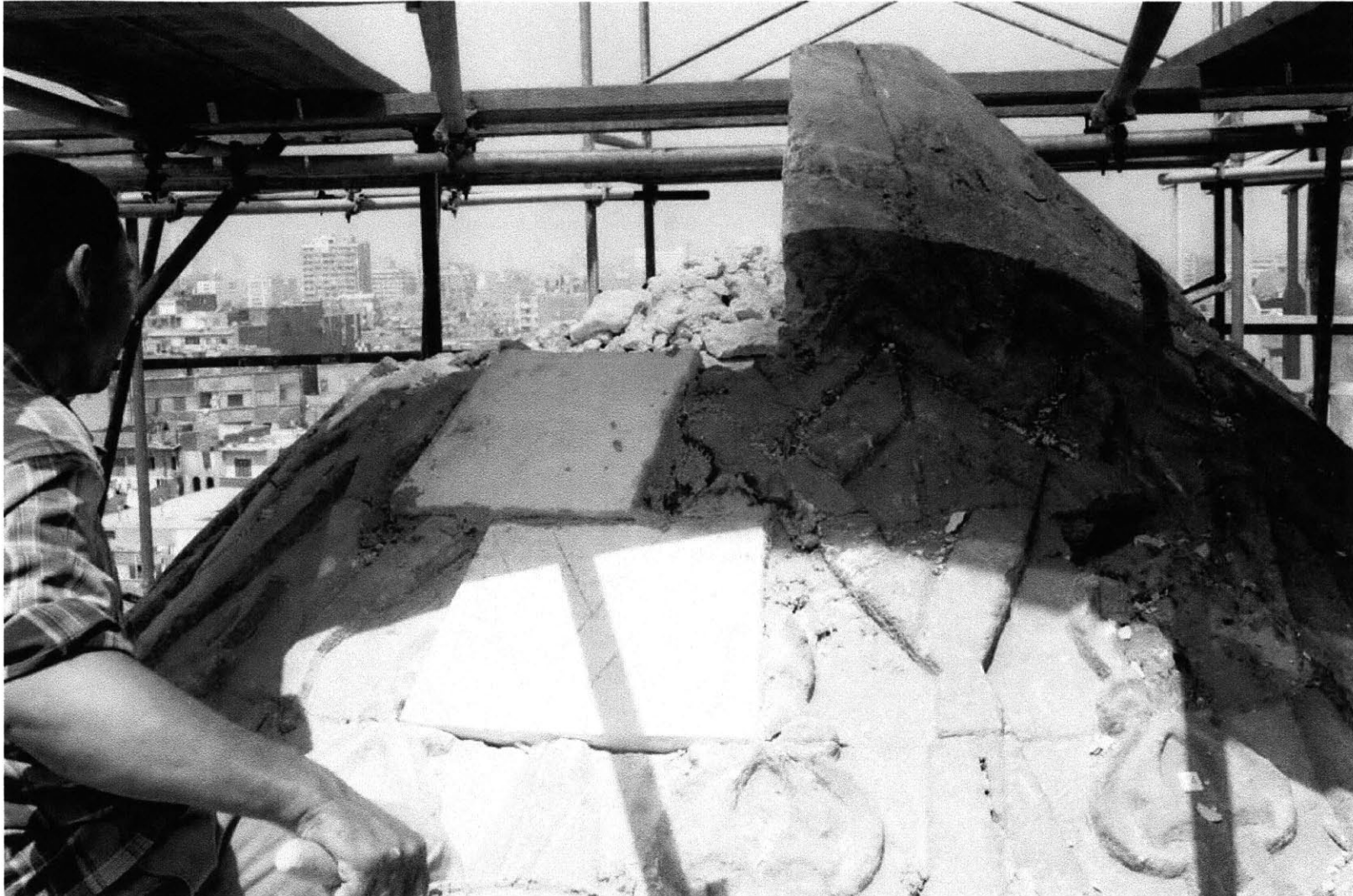
Fig 2.30 This picture of the restoration works proves that at least the first four upper courses are constituted by two layers, the external one are stone blocks of 15-20 cm of thickness. Picture courtesy of the Aga Khan Trust for Culture.
