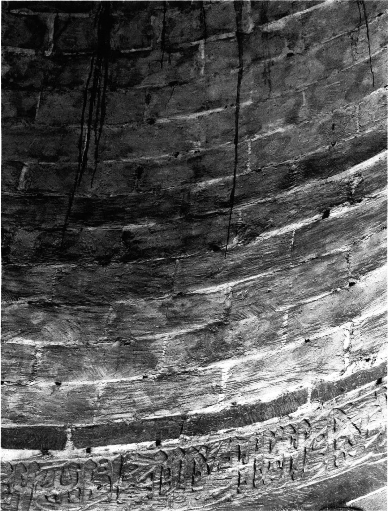
Fig 2.28 Detail of the dome from the interior . Wood pegs used during construction are visible in correspondence of the joints.
