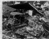
DOZER ALSO HANDLES THE FOURTH AND FINAL STEP —With the bulldozer still in charge, the area is cleaned up. The basement excavation is filled in and the lot is smoothed over. It all looks so easy when man and machine team up to clear the way for the new freeway.
