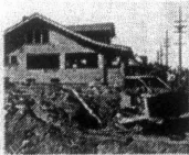
CONTRACTOR PREPARES HOUSE FOR DESTRUCTION —The first step in the house wrecking technique displayed by the District 7 crews as they clear the area for the new freeway by Lake Union in Seattle is shown above. The contractor strikes a cable through the house and attaches it to a medium size bulldozer.
