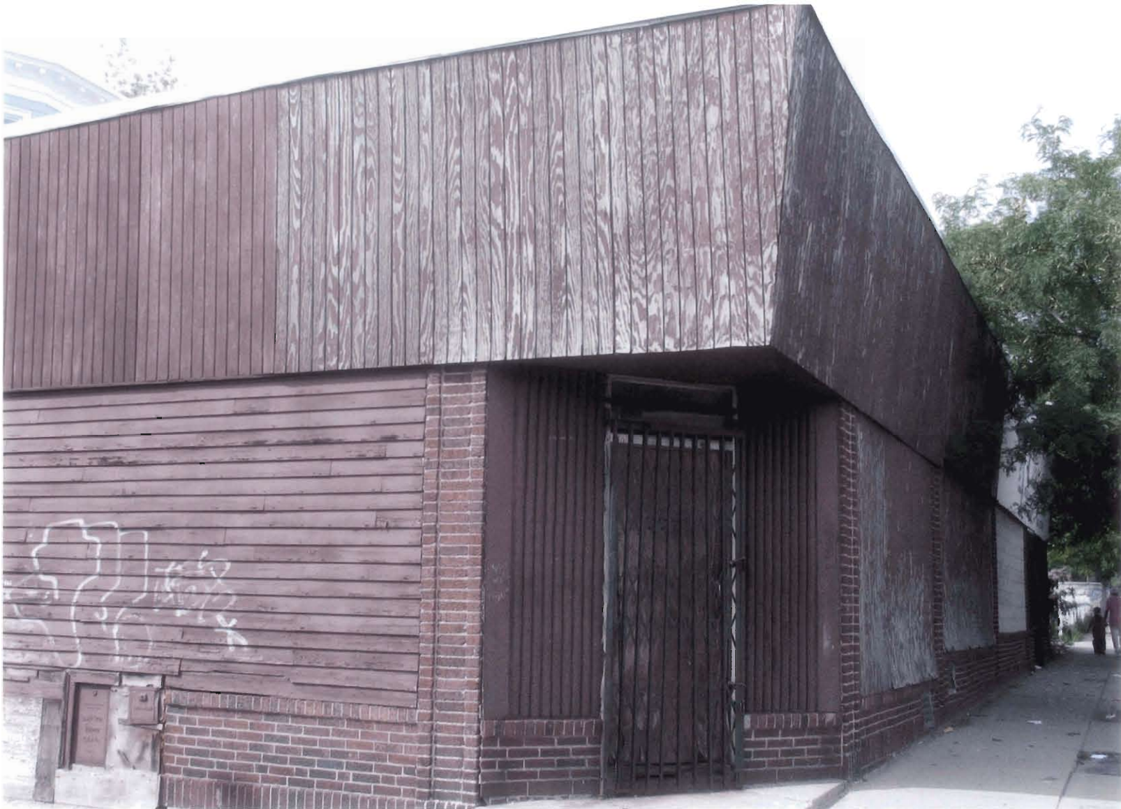
abandoned building, Washington Street
