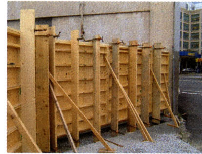
Fig. 70. Image of Formwork 2. 2x8 supports are placed vertically and fixed at top and bottom of the wall.
