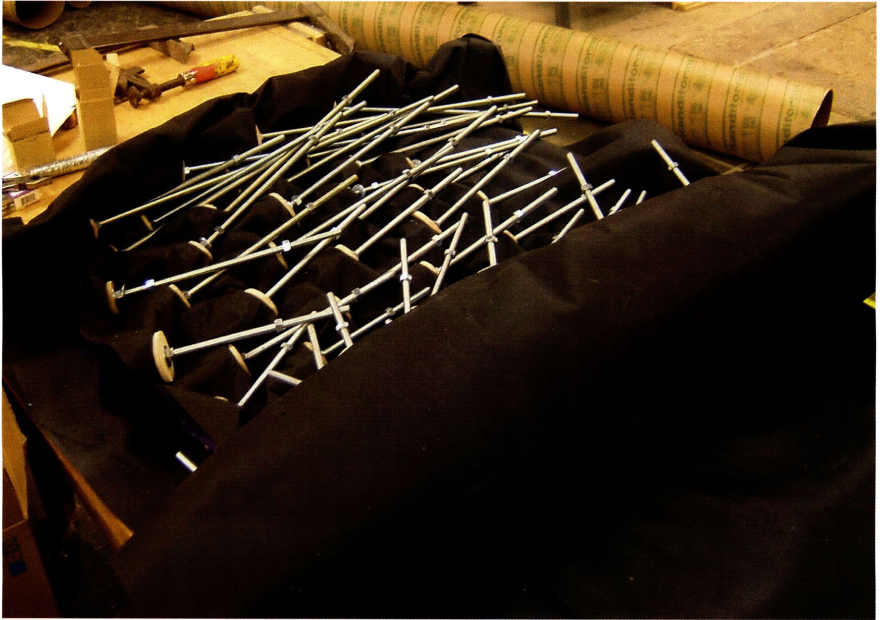
Fig. 156. CONSTRUCTION SEQUENCE 4. Steel rods are attached to the fabric by the foam spacers..
