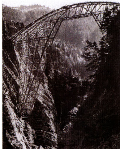
Fig. 11. Formwork/Scaffolding designed to hold only the weight of the arch. Once set, arch became the working ground for the structure above.
