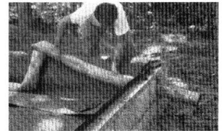
Fig. 28. Tube in a Beam. Shows how air tubes are used to create holes in a beam. (formwork book)
