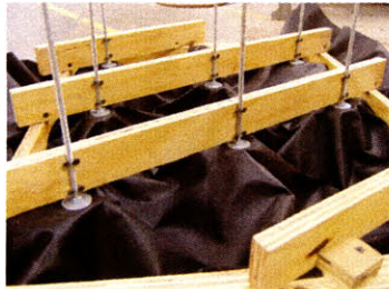
Fabric is hung with slack to allow concrete to generate its own form
