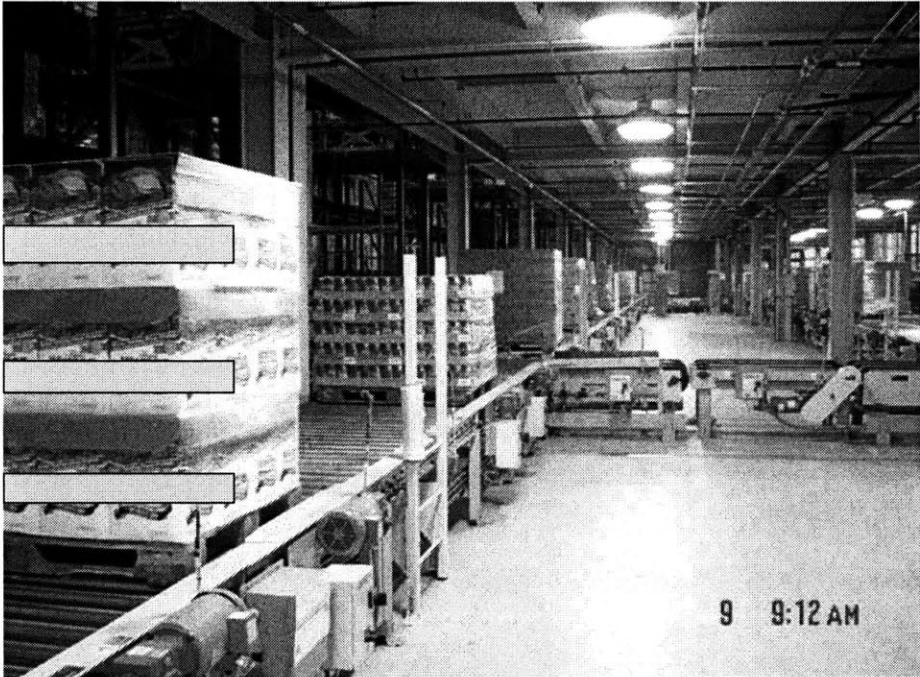
Photo 2 Main Conveyor Loop
