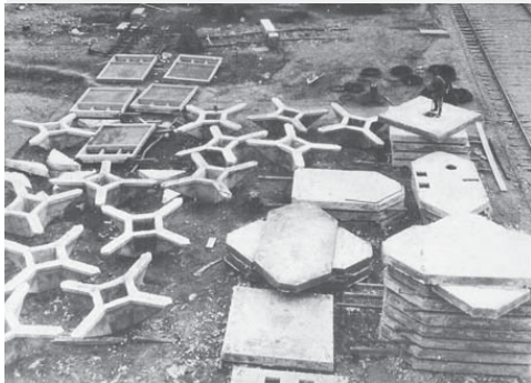
↑ Square and hexagonal floor panels, and cruciform capitals were cast on site.
