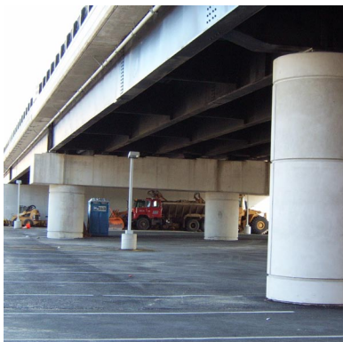
Various uncoordinated support conditions for Summer Street Bridge, 2006
