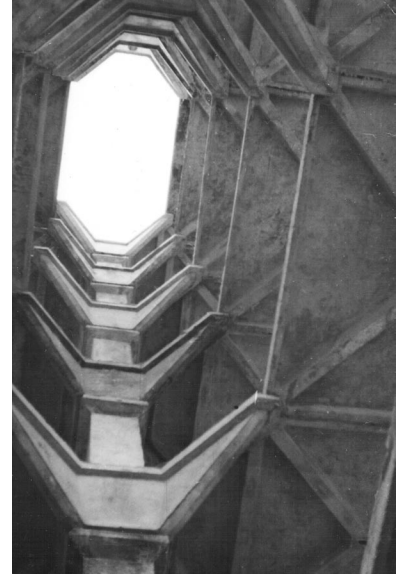
Internal view of capital floor system design by Zalewski with tapered column capital arms and open light wells [Zalewski 2006]
