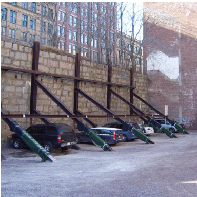
Steel reinforcement along unstable seawall next to Summer Street Bridge, 2006
