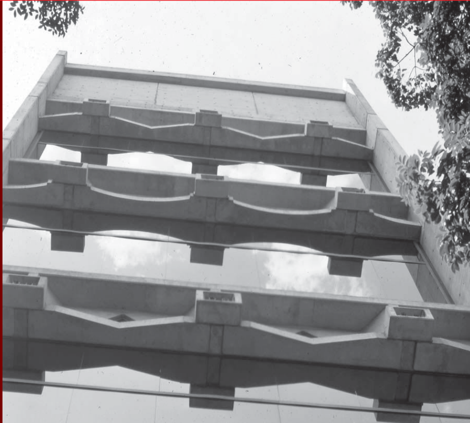
↑ In this view looking upward along the facade, exposed concrete boxes mark the anchorages of the prestressing cables. The indentations of the slabs' edges express the manner in which compressive forces radiate from the anchorages.
