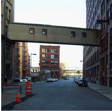
Existing conditions with underground utility repairs underway and trees dying
