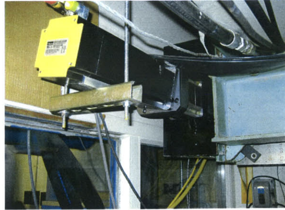
Figure 15. Servomotor assembly permanently attached to the drive system.
