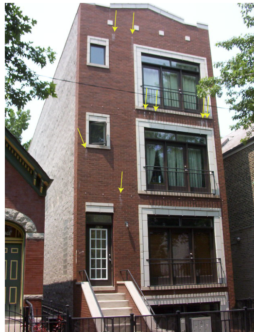
Figure 35. White streaks, indicated by the yellow arrows, can be seen on the front facade of this recently-built three-flat, Ukrainian Village, Chicago. They indicate that faulty construction has allowed moisture to penetrate behind the brick veneer. Also note that small drains (generally lying at the top of each streak) have been installed to drain the excess water.
