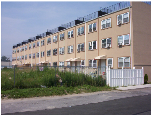
Figure 42. Masonry parapets extend the fire separation party walls above the cornice line on a row of three-family houses, Far Rockaway, Queens. This adds to the cost needed to bring a three-family house in New York City into compliance with the local building code. The local requirement that the ground-floor units be wheelchair-accessible raises the building height to the minimum where a parapet is required.
