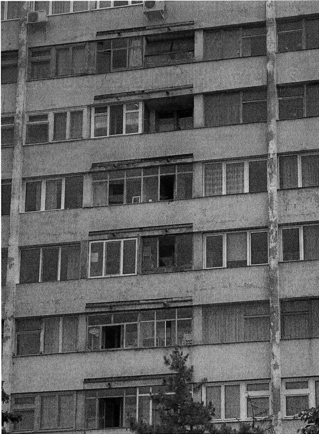
Fig. 3. Floreasca Towers in their present, dilapidated, state. Photo by author, 2004.
