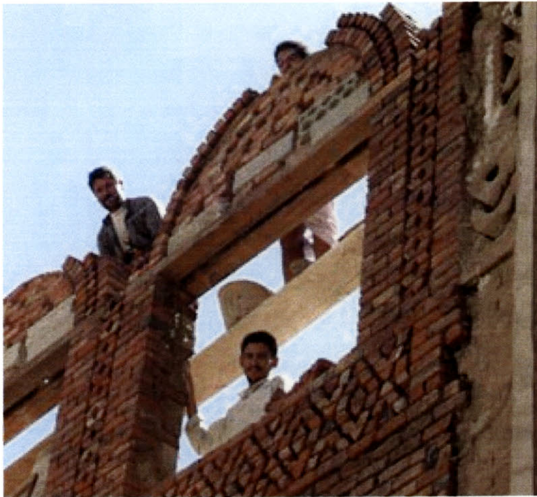
Figure 17 Construction of an upper story in the eastern part of the old city. Traditional-style brickwork, executed with half bricks, is applied as veneer to concrete block walls – a common solution that is usually approved by inspectors.
