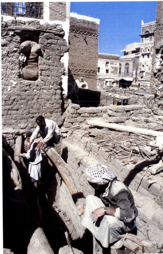
Figure 51 The restoration of a caravansaray near Bab al-Sabah that houses migrant workers, sponsored by Oxfam. Restoration directed by Abdullah al-Hadrami.
