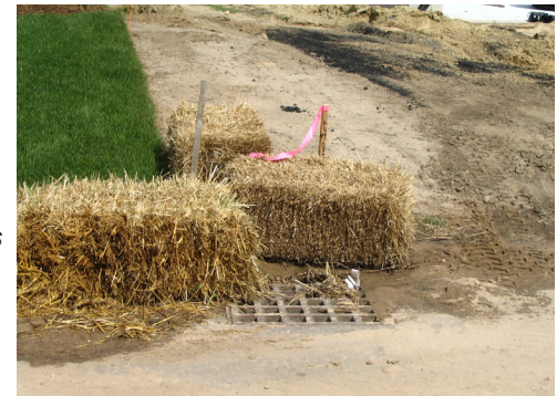
(clockwise from top left) Moore marks narrow limits of clearing, creating a rustic and established feeling to new roads; silt runoff from construction sites can threaten the LID stormwater management system; hay bales block silt from drainage system.
