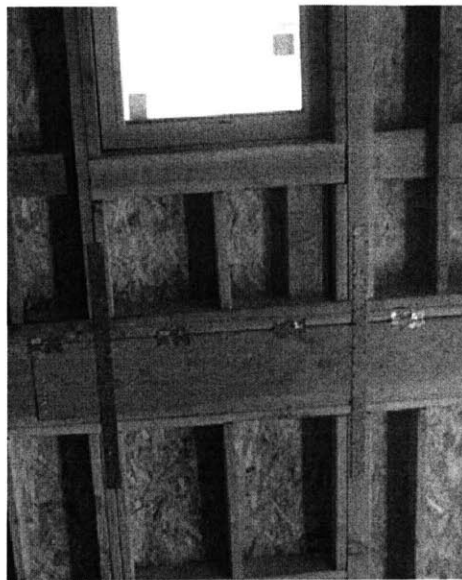
Figure 13: Metal Straps used as Hold-downs from Floor to Floor (Courtesy of Nina Mahjoub, 2007)
