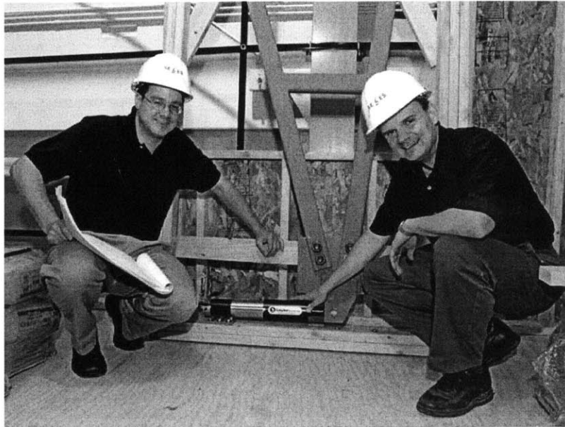
Figure 35: Seismic Damper Installed inside NEESWood Bedroom Wall (University at Buffalo/Parisi, 2006)
