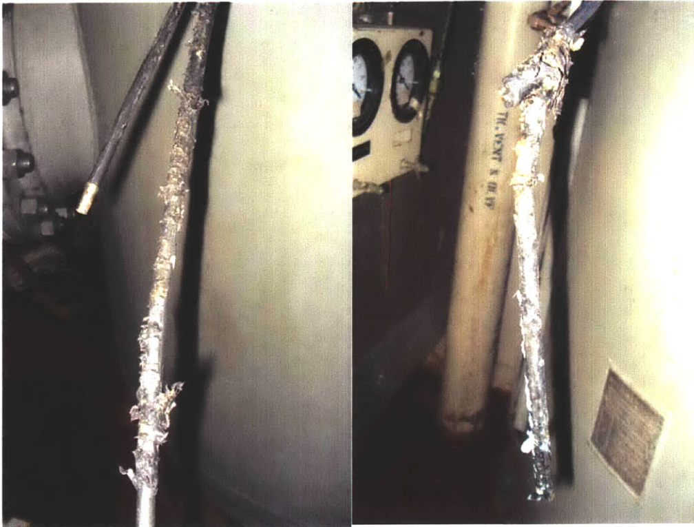
Figure 2-23: Corroded probe coating next to newer probe coating (left); Previous repair insulation blocking control signal while hanging off the tip of the probe (right).
