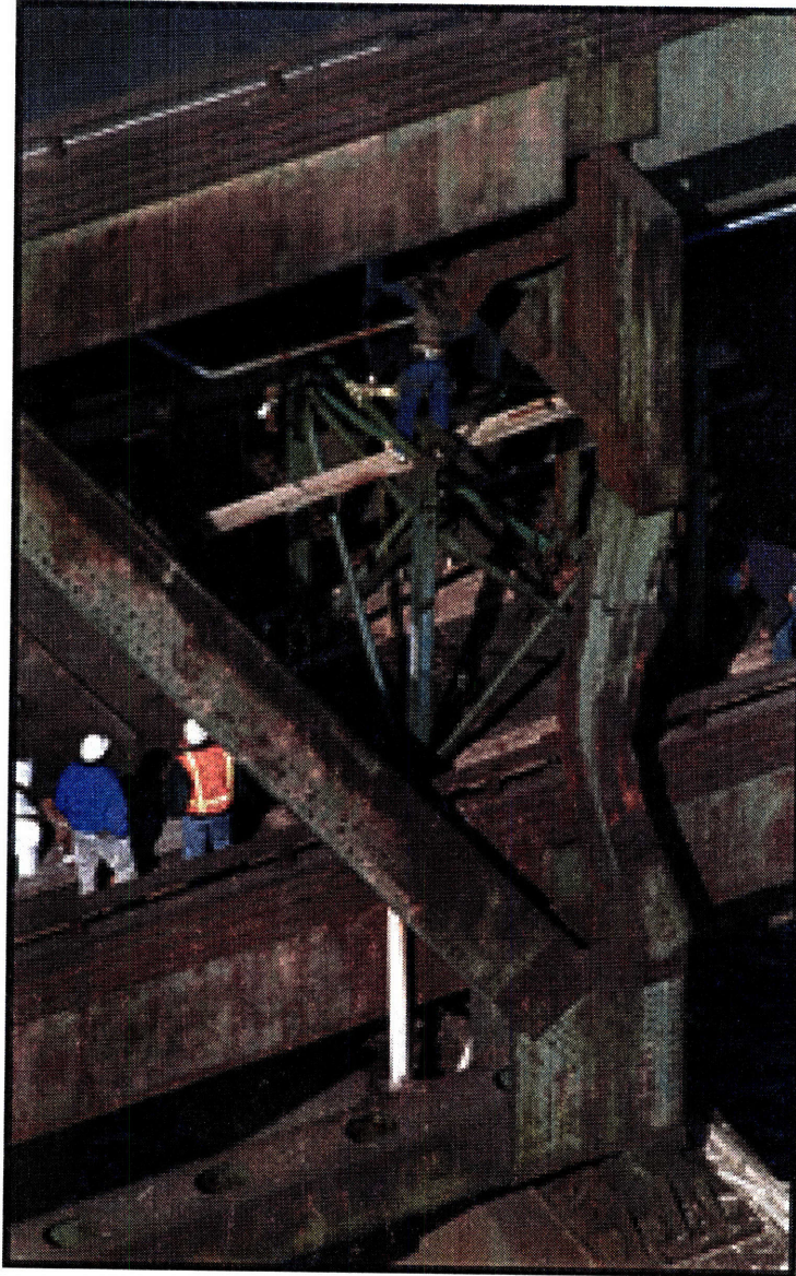
Figure 1-1: Buckling phenomenon in a real, full-scale structure. A 30-foot tall support beam buckled after being hit by a truck in a May 2, 1996 accident on Interstate 93 in Boston, Massachusetts ([8]). The steel beams are used to support the elevated section of the highway at the point where it crosses the Charles River.
