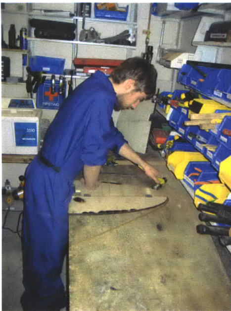
Figure 4.24 The manual formation of the curved brass frame using a laser-cut plywood template.
