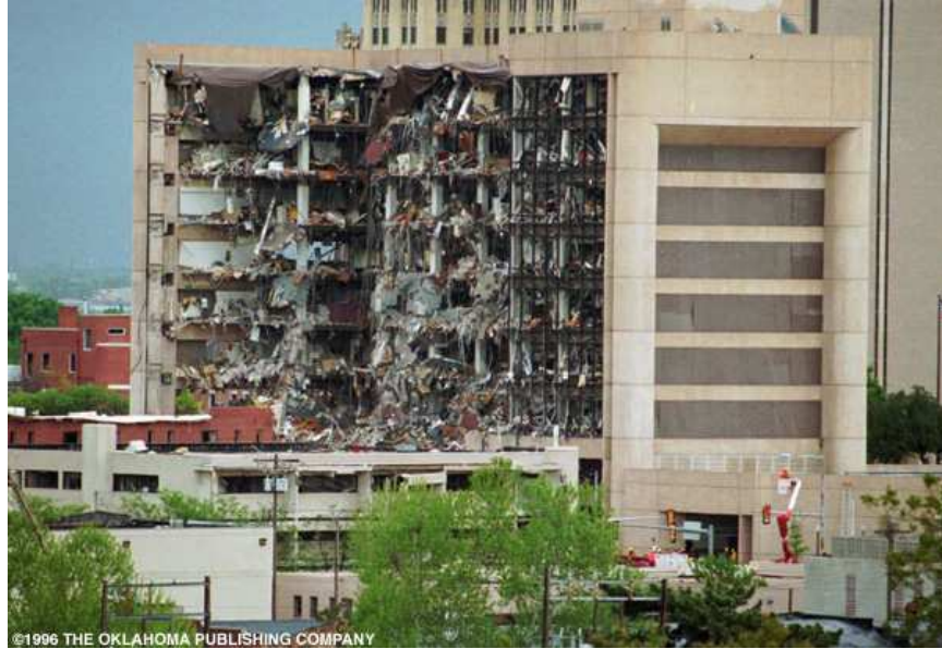
Figure 1-1: The Alfred E. Murrah Federal Building in Oklahoma City, Oklahoma after the terrorist attack of April 19, 1995 [18].
