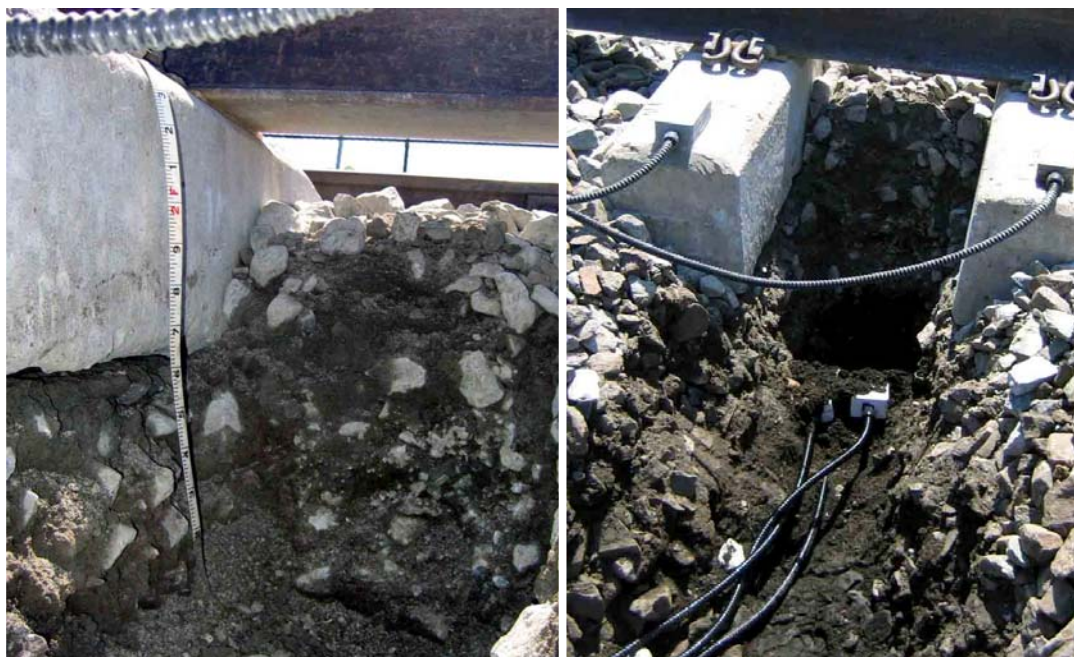
Figure 6-9: a) Fouled ballast between the concrete ties at the problematic area, b) Installation of sensors just below the fouled ballast.
