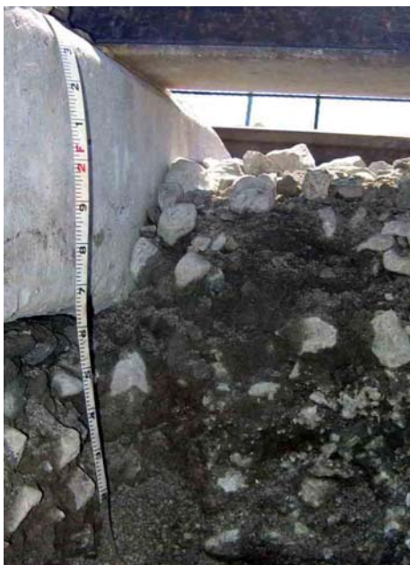
Figure 2-8: The ballast at the problematic mud pumping site is fouled with infusion of subgrade.
