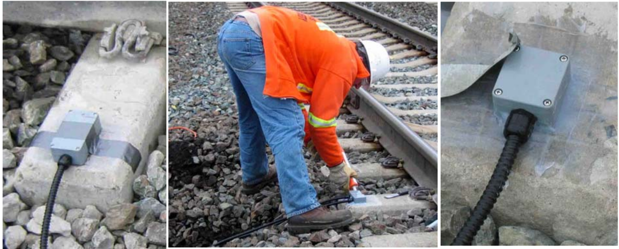
Figure 6-4: a) the epoxy was allowed to harden during the 10 minutes setting time, b) application of silicone spray to protect weathering of epoxy, c) final working stage of the sensor.
