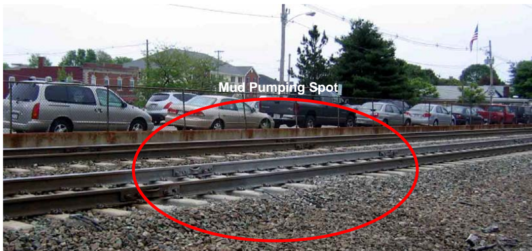
Figure 2-2: P2 - Mud Pumping Site at Mansfield. The mud pumping spot is visibly marked by white patches on the rails and concrete ties.
