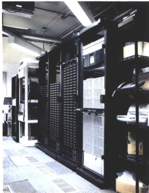
Figure 3.8: Several hundred terrabytes of HSP data is stored on dedicated hard drives, which occupy the four racks in the center.
