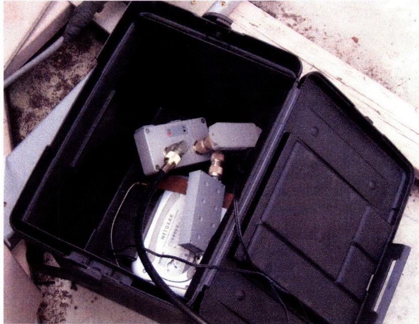
Figure 6-19: Transmitter electronics housing on top of Green Building
