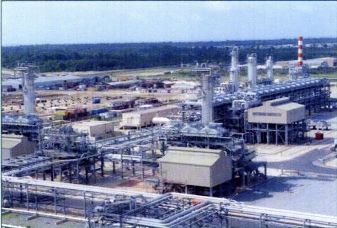
Figure 8: Nigeria LNG Plant in Bonny Island (NLNG, 2008)
