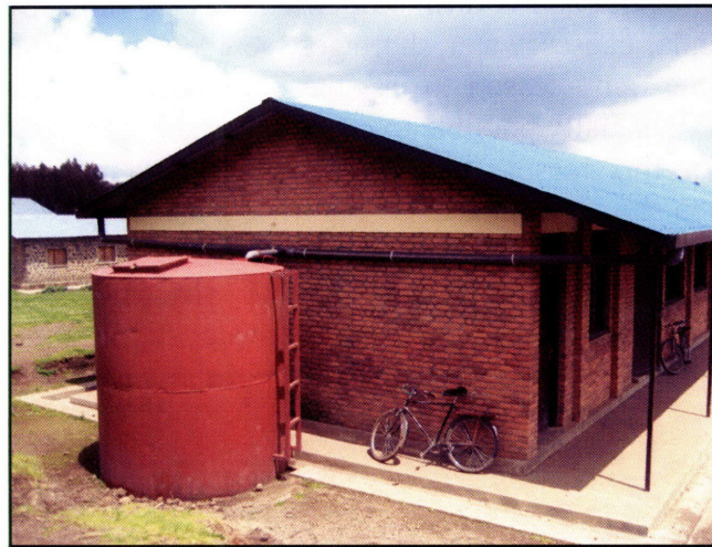
Figure 2-1 : Rainwater Harvesting System at a Rwanda Primary School (2007)
